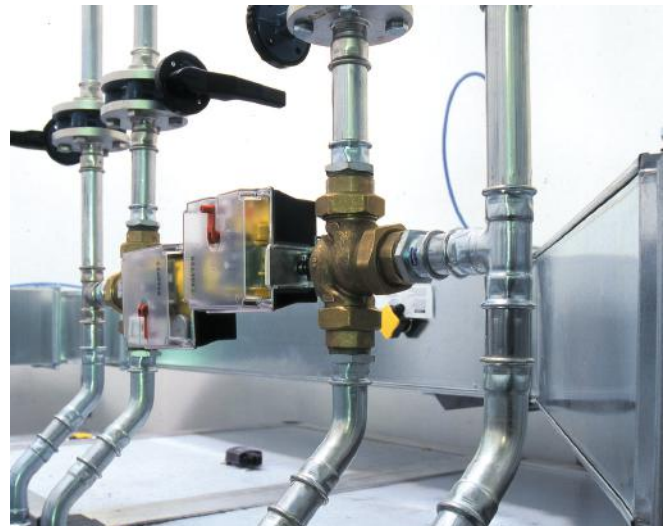
Figure 22 - steelPRES - refrigeration (closed circuit)
